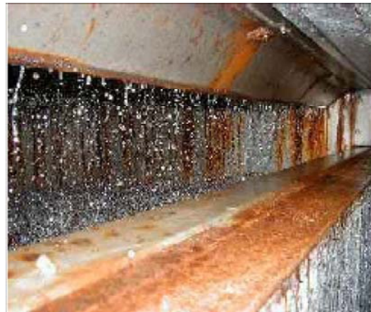
Figure 2. Corrosion damage to the air supply channel of a large auditorium by LiCl solution aerosol
